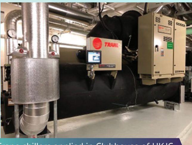
Trane chillers applied in Clubhouse of HKJC
